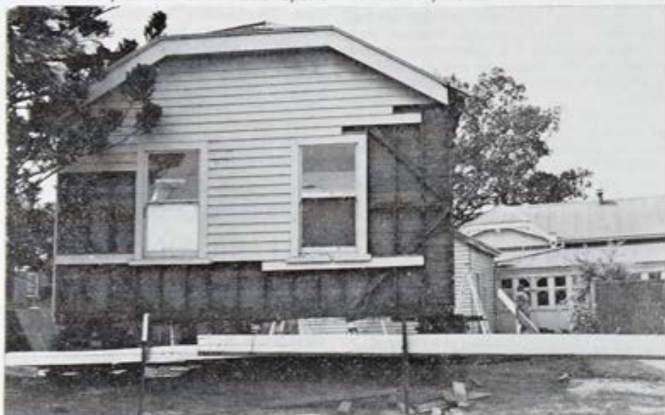
A wing of the original 'Warrinn' boarding house, ready for removal to Campbell House.
